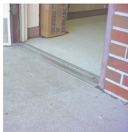
Be careful of uneven surfaces.
